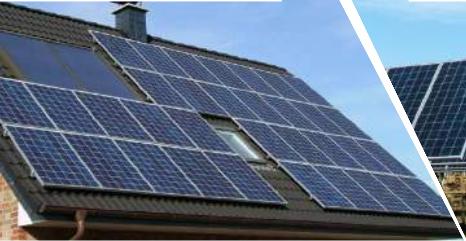
Solar Roof Top System
